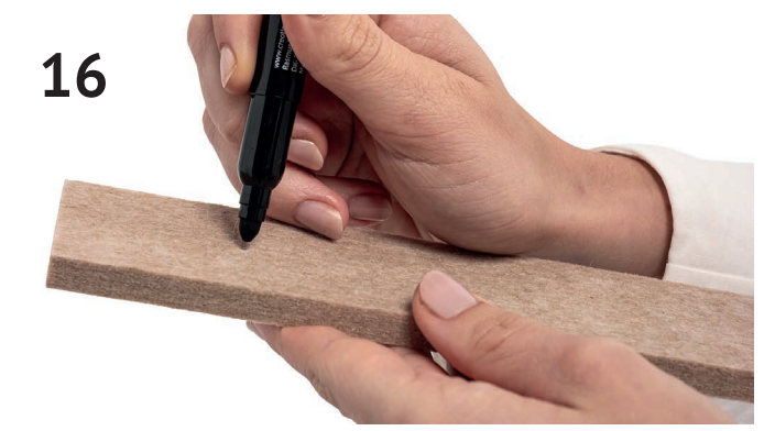
16 Use a marker to mark the drilling points on the felt spacer
